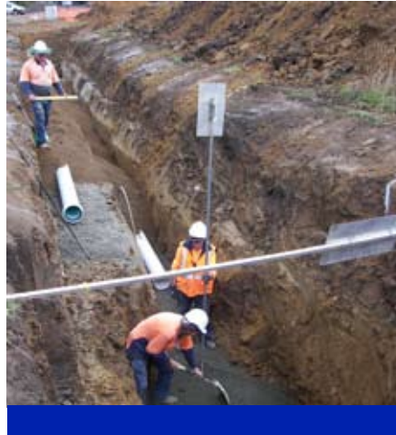
New pipes being laid along Sale Street as part of the upgrade to the Huonville water scheme.
